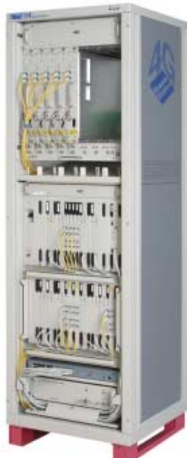
Base station transceiver (Transmitter only)
